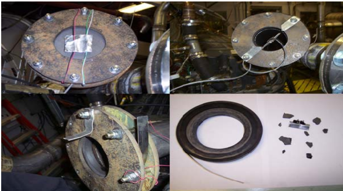
Figure 10 Pressure Relief Valve and Its Burst due to Backfire
