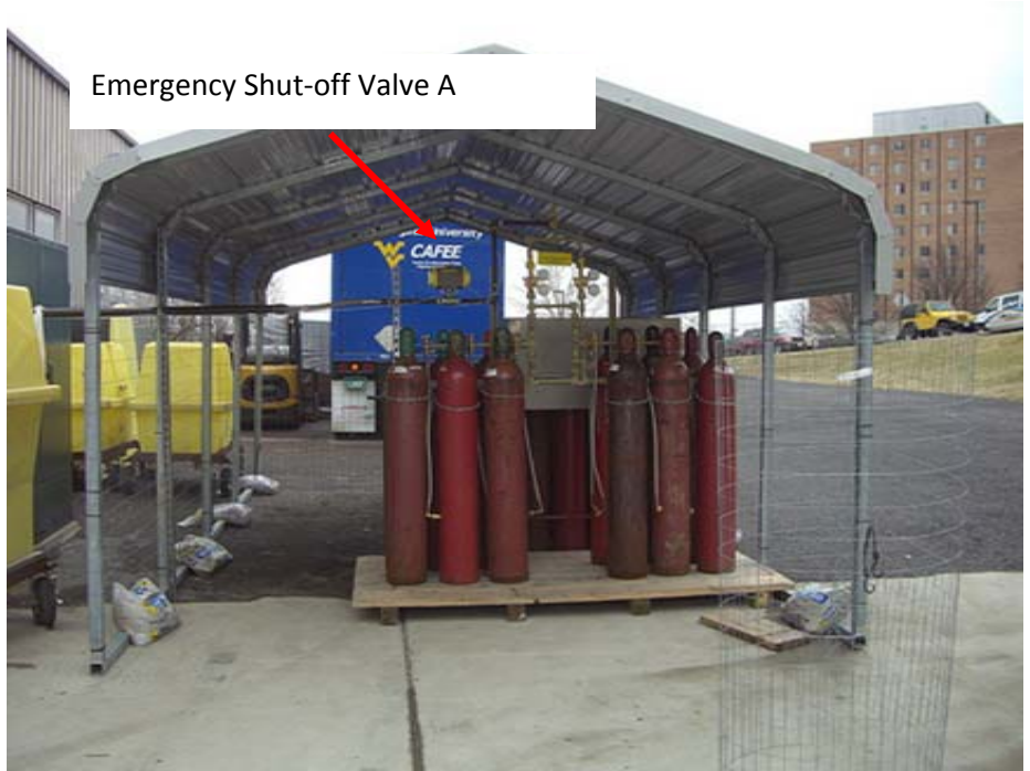
Figure 7 Hydrogen Station with Pressure Regulation Module and Emergency Valve A
