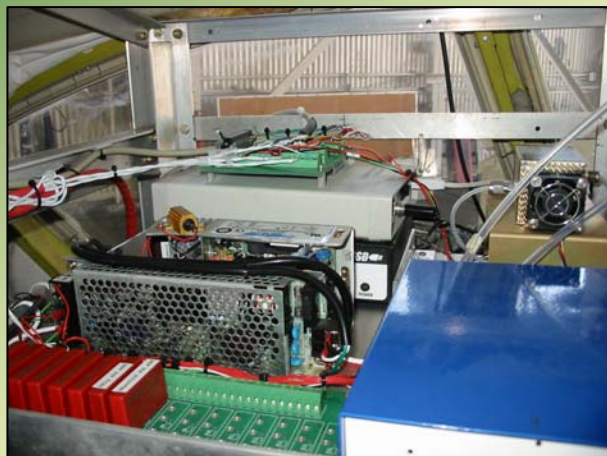
Left: Data system and power supplies
