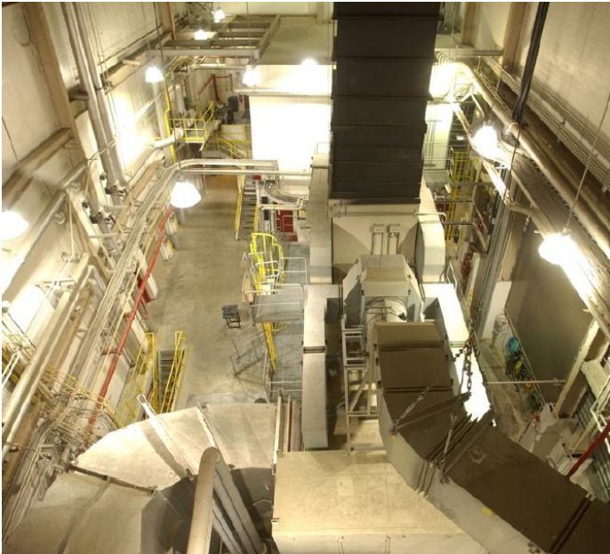
CHP plant facing east, looking down on combustion turbine package from heat recovery steam generator.
