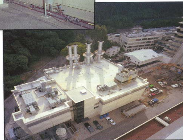
(Right) Aerial photo of the UCSF Central Utility Plant including the gas turbine cogeneration plant and emergency standby diesel generator sets.
