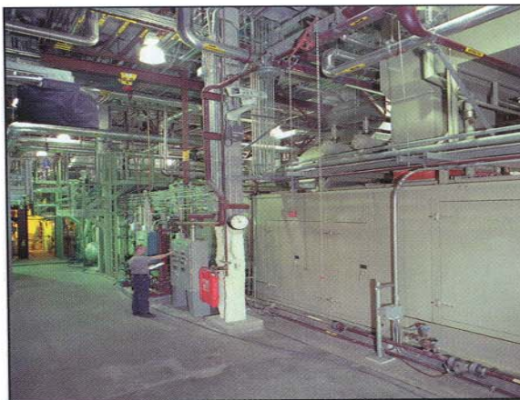
(Left) One of two Solar Taurus 60 gas turbine gen-sets at the UCSF medical complex in a cogeneration application. Each unit produces 4.8 MW output driving an Ideal generator. A steam turbine generator set is also included as a combined-cycle unit, giving a total plant capacity of 12.1 MW.
