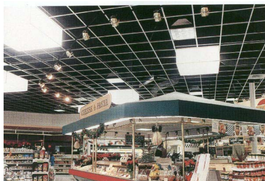
Skylights provide daylighting in a supermarket
