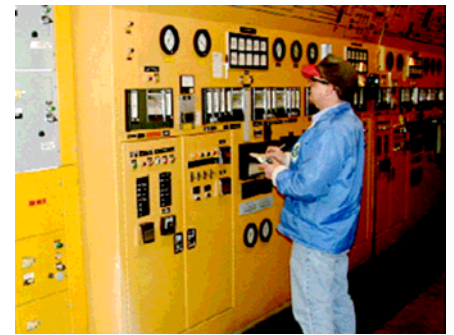
Digester controls at a wastewater treatment plant
