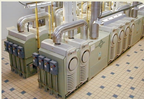
Far left, absorption chiller provides building cooling using microturbine exhaust heat at Harbec Plastics.
