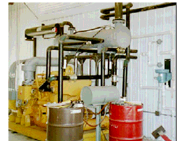
Digester engine with heat recovery system
