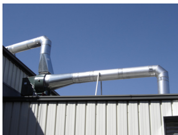
Microturbine exhaust ducting
