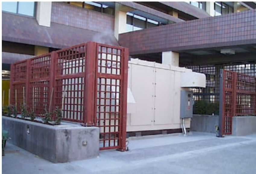
PC25C Fuel Cell Power Plant in operation providing 200kW to corporate data center at ChevronTexaco Park
