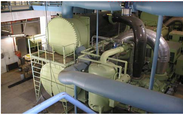
Figure 3. One of UT-Austin's 5,000 ton electric chillers. Source: UT-Austin
