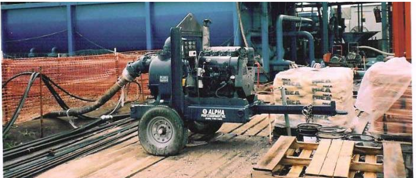
Figure 4. Slurry Pump Used for Pit Circulation, Fluid Transfers, etc.
